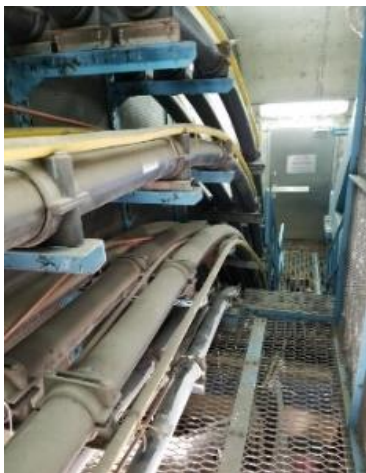
View of Compartment A of the cable bridge, from inside the bridge and looking towards Kwong Yip Street entrance, showing the cable racks on 132kV cables.
