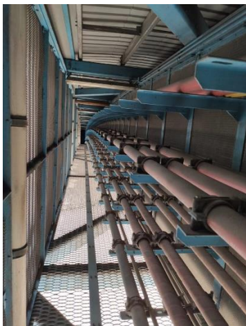
View of Compartment B of the cable bridge, from inside the bridge and looking towards Kwong Yip Street entrance, showing the installation of the 11kV and the disused 132kV now drained oil filled cables (lower layer).
