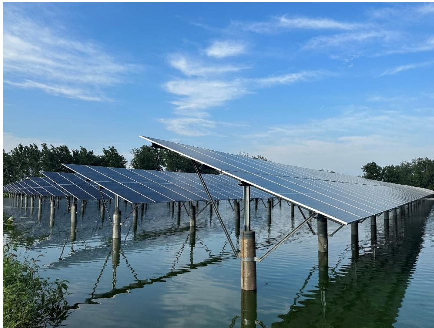
CLP's Jiangsu Yangzhou Gongdao Solar Power Station.
