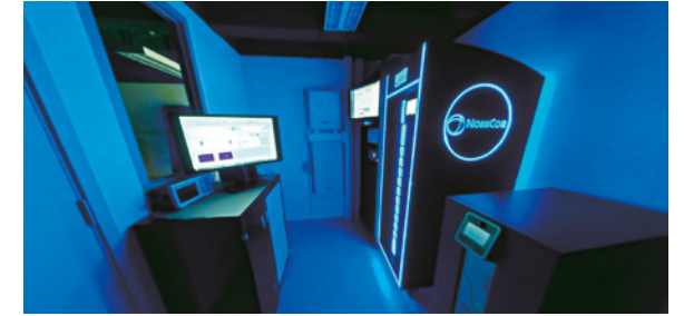
智能電網運行中心配備實時數字仿真系統和功率硬件在環測試平台。 Smart Grid Operation Centre is equipped with Real Time Digital Simulator and Power Hardware-in-the-Loop testing platform.
