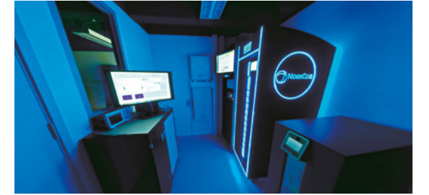
智能電網運行中心配備實時數字仿真系統和功率硬件在環測試平台。 Smart Grid Operation Centre is equipped with Real Time Digital Simulator and Power Hardware-in-the-Loop testing platform.
